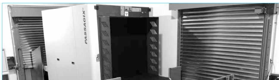
Shutters anti-intrusion – fire doors
