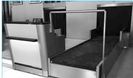
Odd-size baggage check-in conveyors
